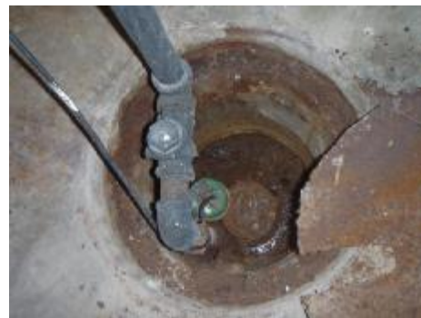
#39 Old rusted sump pump. It works
