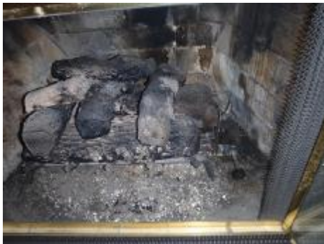
#31 It needs cleaned before use. The gas supply line needs a shut off installed
