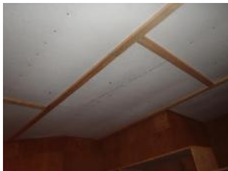
#23 Ceiling should be half inch drywall with taped seams to make a smoke-fire barrier between house and ga
