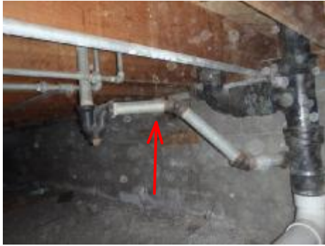
#49 Galvanized drain lines
