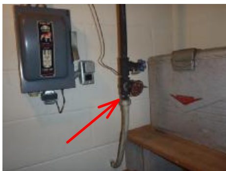
#44 Whole house water shut off
