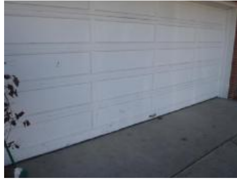
#2 Minor painting is needed
