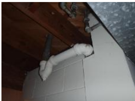
#40 Galvanized drain and water supply lines
