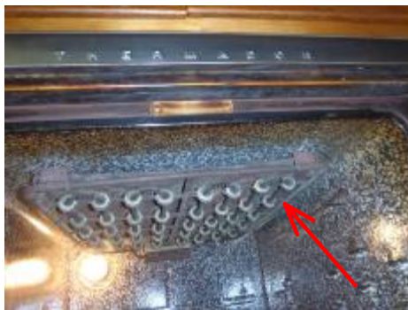
#38 Oven heat elements are exposed and will shock if touched.
