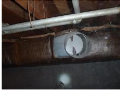
#50 Heat for crawl space
