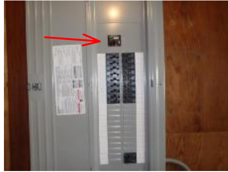
#26 200 amp main breaker
