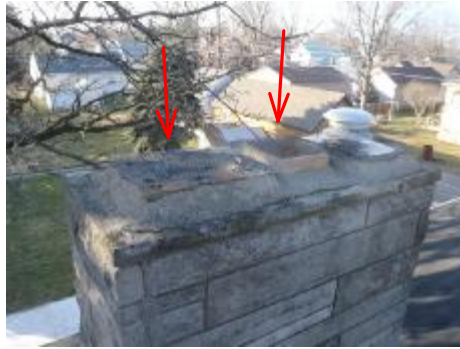
#14 Recommend a flue caps be added.
