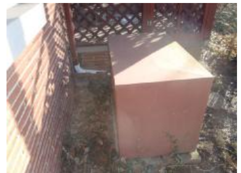
#9 Old AC not inspected
