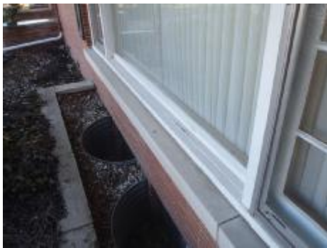
#4 Minor painting is needed
