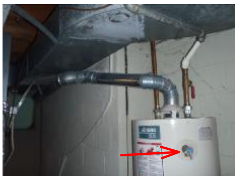
#43 Discharge pipe needs to be extended to approximately 6 inches from the floor
