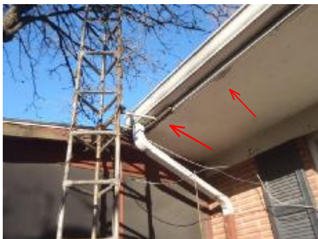
#7 Needs scraped and painted
