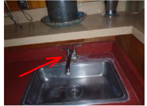
#27 Loose. Hot does not work
