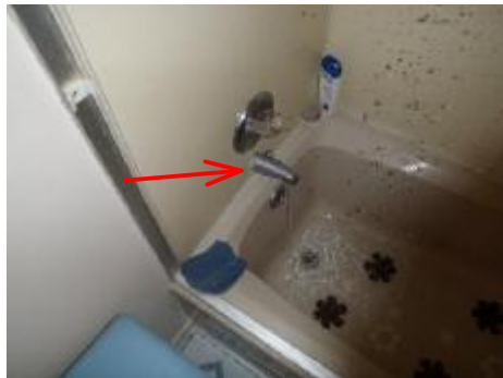
#44 Shower diverter does not direct all of the water to the shower head.
