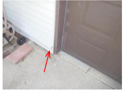
#3 Loose by garage door
