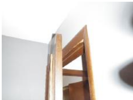
#47 One door needs trimmed at bottom, One needs trimmed at top.
