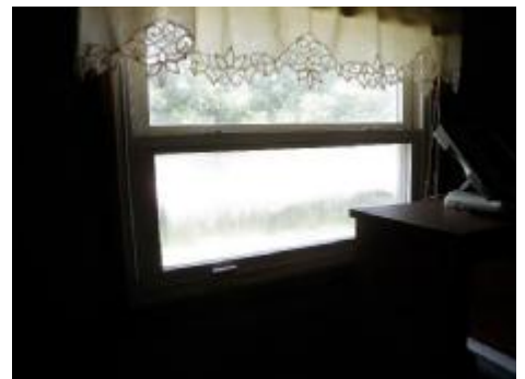
#48 Double paned window has lost the thermal seal and is fogging over X 2
