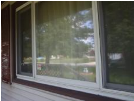
#4 Double paned window has lost the thermal seal and is fogging over.
