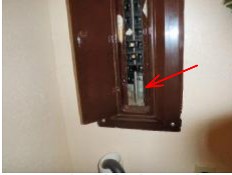
#37 Breaker blanks need to be installed for safety.
