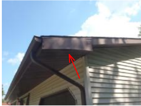
#2 Loose on south end
