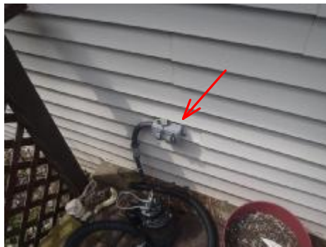
#17 Recommend Exterior outlet be GFI protected
