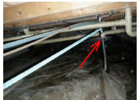
#60 Whole house water shut off
