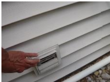
#20 Outside baffle is not to have a screen or grid on it that will restrict air or lint.
