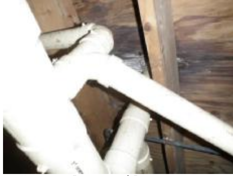
#62 Below toilet. Past leak
