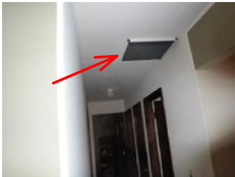
#43 Old furnace filter
