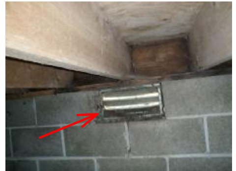
#54 The screens on the vents are torn/ missing and need repaired to keep out mice.
