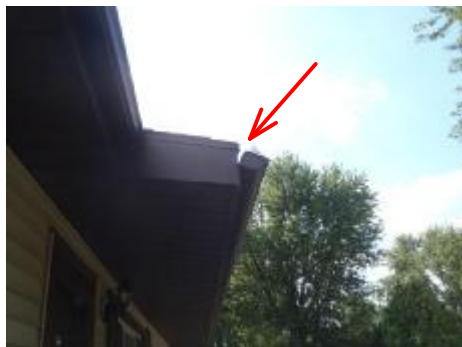
#8 Loose above front porch
