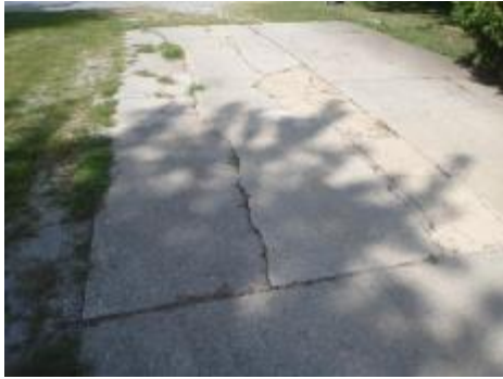
#1 Heavy cracks in surface
