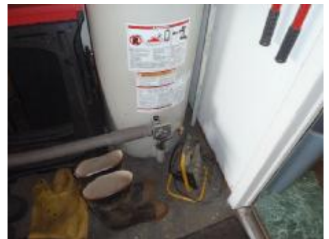
#33 The water heater needs to be 18 inches above the floor.
