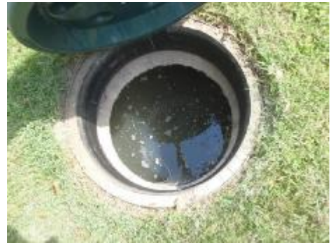
#6 Cover for septic needs to be secured.
