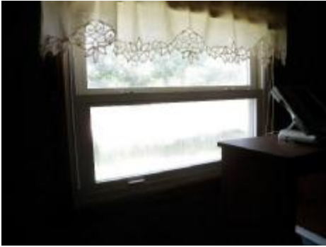
#49 Double paned window has lost the thermal seal and is fogging over X 2
