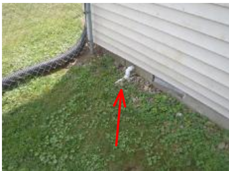
#7 Sump pump discharge
