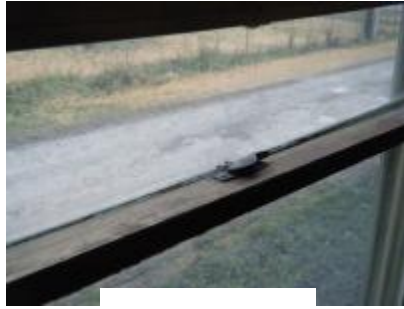
Window would not lock
