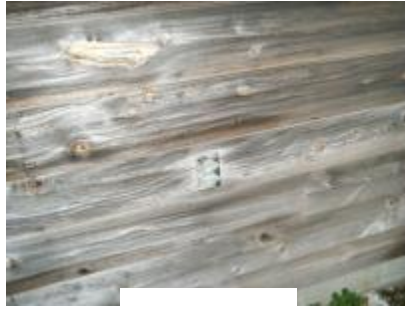
Outlet did not work
