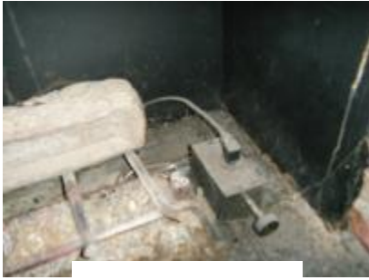
Clean fireplace and gas log
