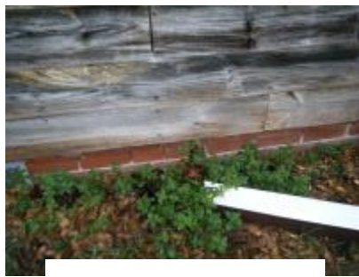
Minor tuck pointing recommended
