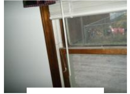
Broken window suspension
