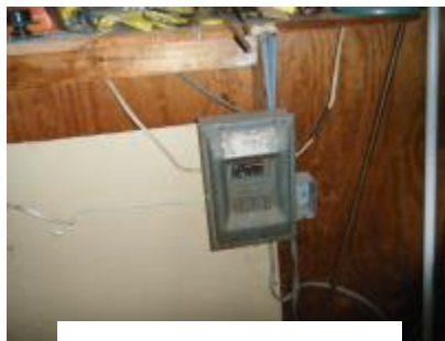
120 volt 20 amp service to garage
