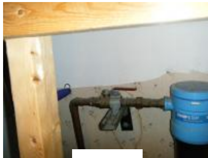
Water shut off
