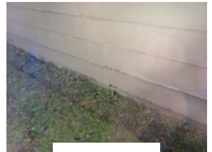
Rotted siding at bottom
