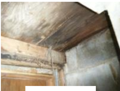
Past leak in wood storage
