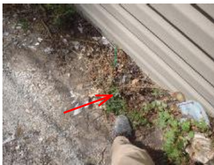
#23 Ground rod should be buried
