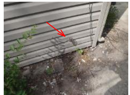
#21 Not frost proof. Shut off inside
