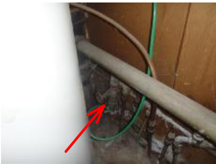
#52 Whole house water shut off
