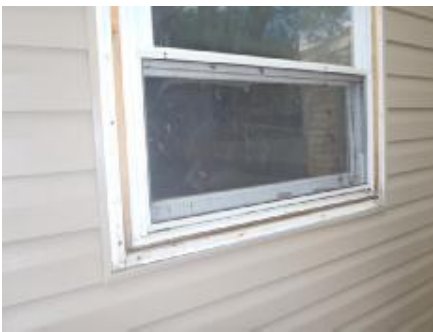
#19 To be replaced
