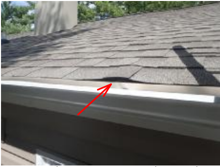
#1 Drip edge aluminum is buckled up in several areas. It should be nail down to look better
