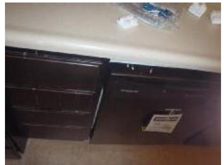
#48 Needs fastened to counter. Inoperative at time of inspection
