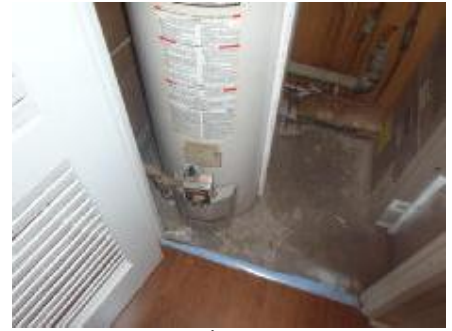
#51 Gas is off Not inspected
