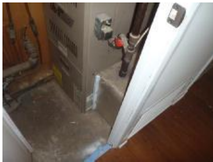
#53 Gas is off. Not inspected
