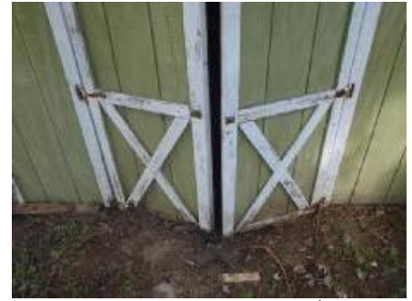
#15 Doors need repaired
