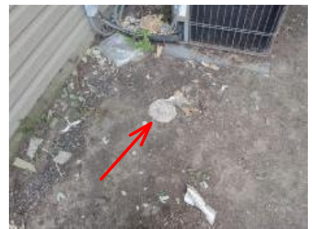
#18 Main sewer clean out
