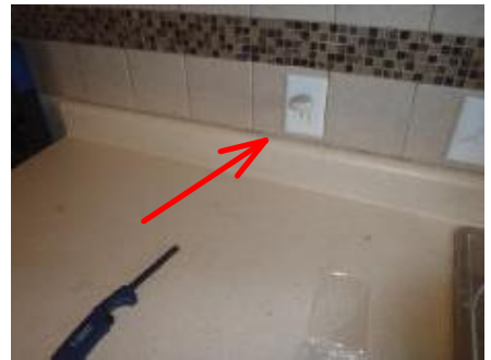
#45 All counter outlets need to be GFI protected
