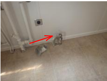
#40 Cap gas line
