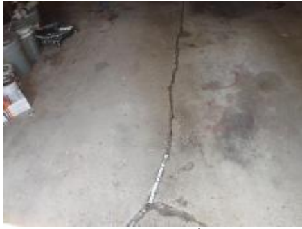
#26 Large cracks in garage floor
