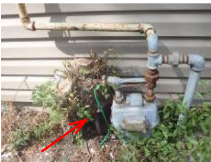
#22 Whole house gas shut off
