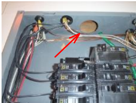
#44 Unused holes need plugged.
